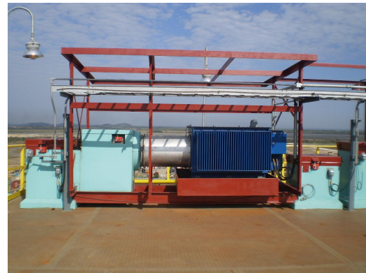
Fig. 1 Coromax HV oil tank
