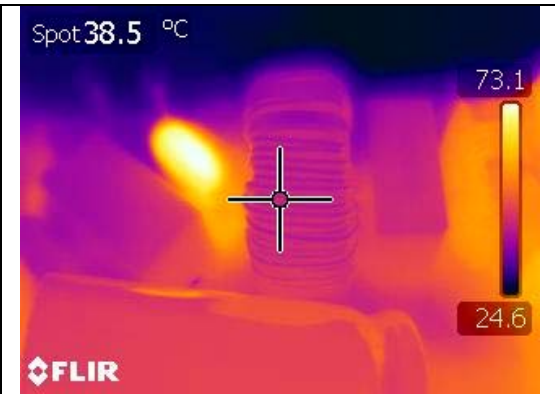
Figure 64 - Common Mode Choke (L1), 230 VAC Input, 100% Load, Room Temperature.
